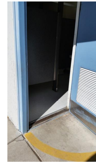
Photo -2 Entrance into restroom does not meet accessibility standards.
